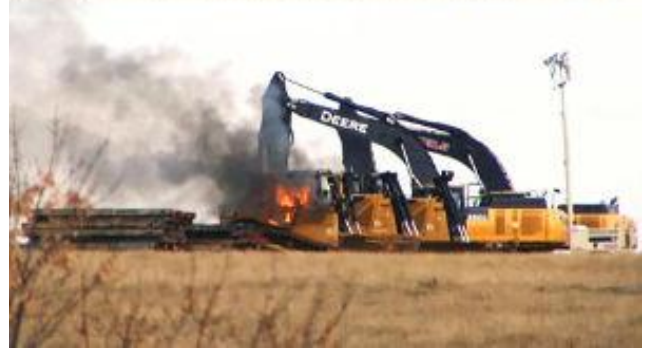
Sabotage of DAPL pipeline construction
