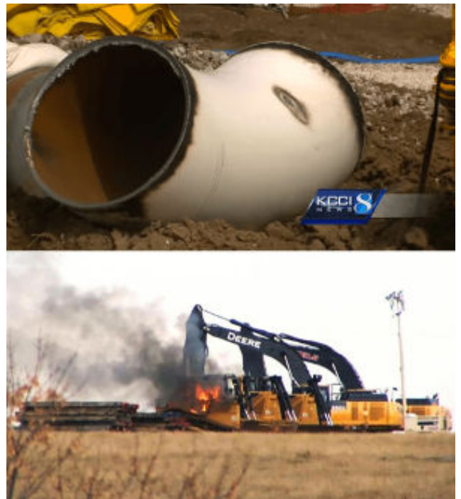
Sabotage of DAPL pipeline construction
