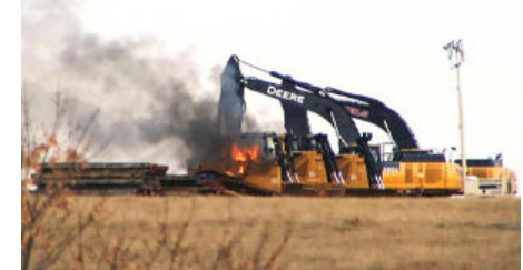
Sabotage of DAPL pipeline construction
