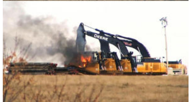
Sabotage of DAPL pipeline construction
