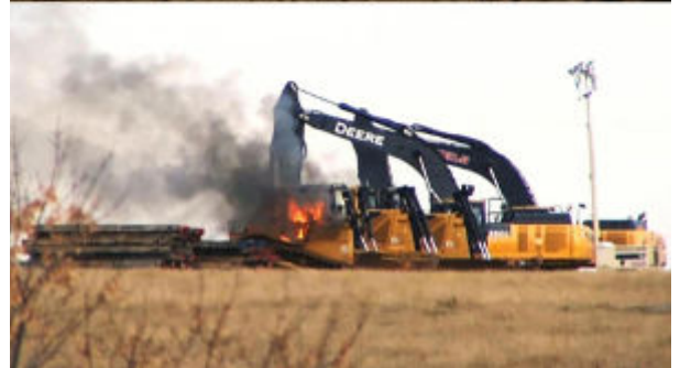
Sabotage of DAPL pipeline construction
